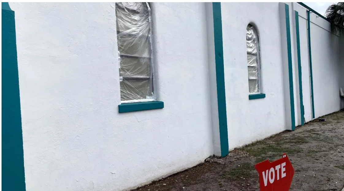
Victory Baptist Church, a temporary polling place in Tampa, Florida during the 2024 presidential election, had plastic covered windows due to damage from Hurricanes Helene & Milton. Crist .
